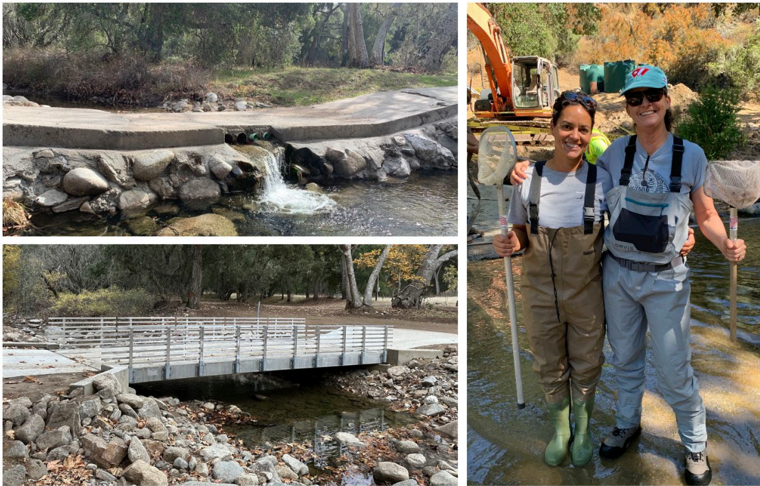
The original stream crossing (top left) and the new Finch Creek bridge (bottom left). Jen Hunter (Hastings) and Bev Chaney (MPWMD), preparing to help move young steelhead out of the project area (right).
