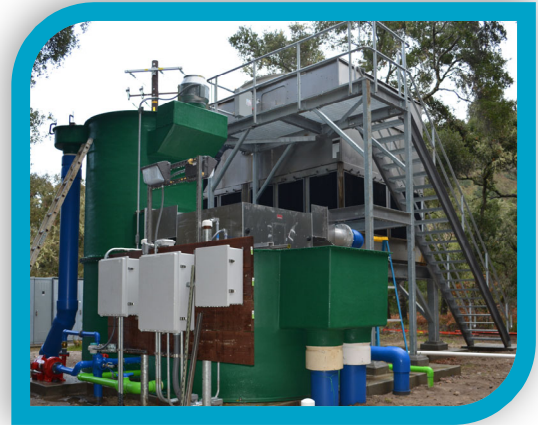
New construction at Sleepy Hollow Steelhead Rearing Facility. When the upgrade is completed the facility will operate during periods of extreme drought or high flows and should be operational for the 2020 fish rescue and rearing season.
