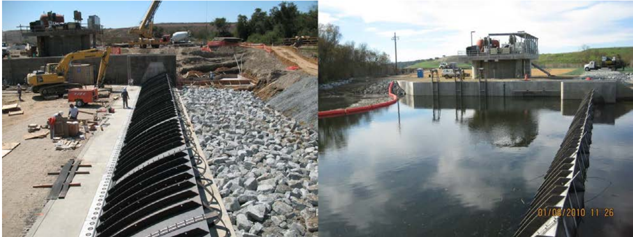
Figure 2-8 Obermeyer Gate at Salinas River Diversion Facility
