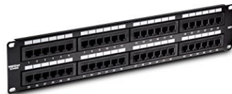
2 48 Port Patch Panel
