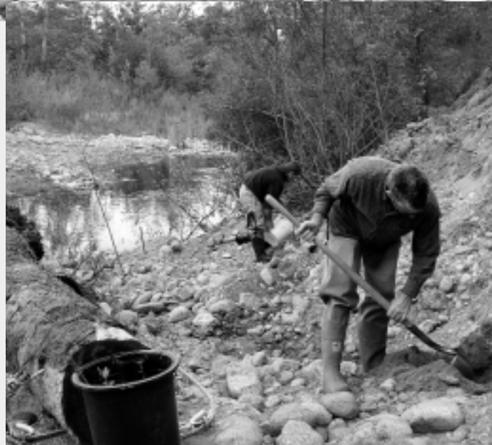
Installation of a large wood habitat structure near deDampierre Park in Carmel Valley Village (pictured: Mark Bekker and Matt Lyons, MPWMD)
