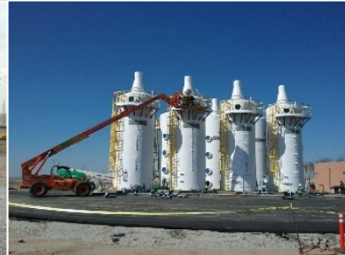
Fresno WWTP Odor Control Facility
