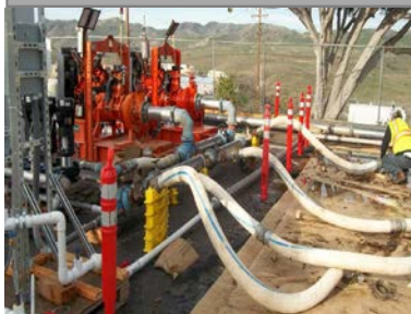
DB Potable Water Storage Tank Pipelines
