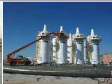
Fresno WWTP Odor Control Facility
