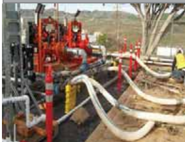
DB Potable Water Storage Tank Pipelines
