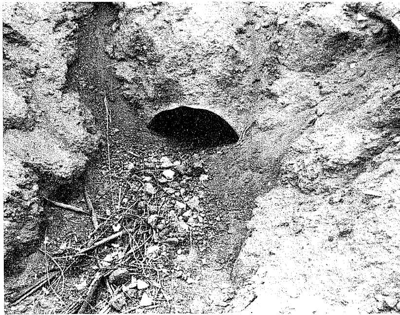
TYPICAL SEDIMENTATION OF CULVERTS ON TRIBUTARIES TO CANYON DEL REY CREEK
