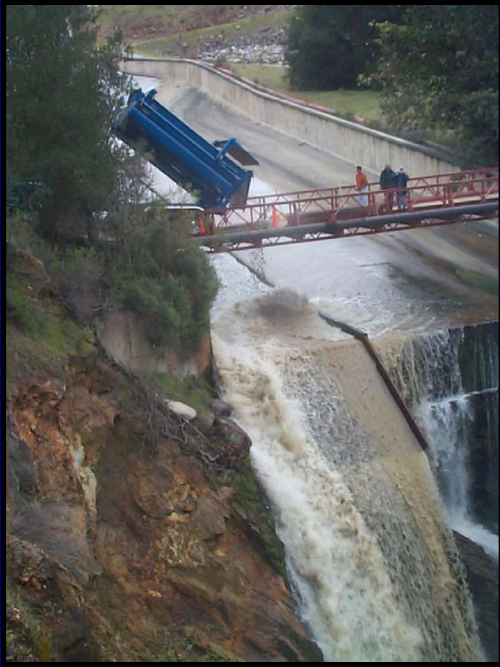
Placing spawning gravel through the bridge at the Los Padres Dam spillway.
