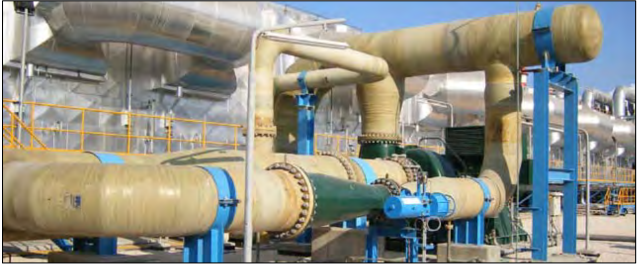
Example of above-grade FRP piping
