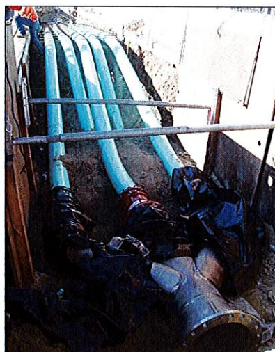
Fusible Sweeps™ over Bridge
