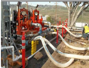
DB Potable Water Storage Tank Pipelines
