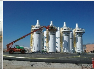
Fresno WWTP Odor Control Facility
