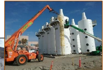
City of Fresno WWTP Odor Control Plant, Fresno, CA
